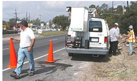
Photo courtesy of the U.S. Army Corp of Engineers. This picture shows actual disaster site work conditions and may not illustrate proper safety and health procedures.
